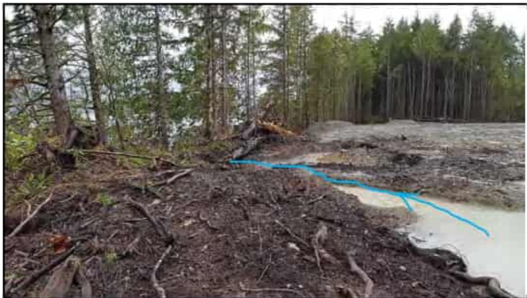
Photo 10: Cleared section of site within 30m foreshore buffer. 30m foreshore riparian buffer to be re-established.
