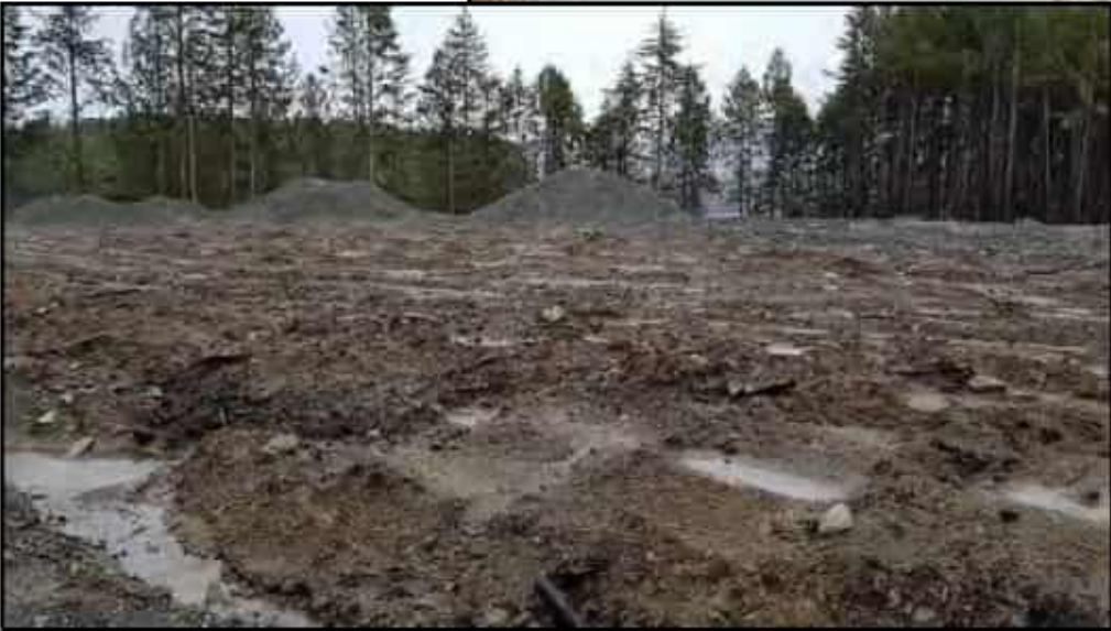
Photo 9: 2017 Image of cleared and grubbed section of site in northern half of property. Portion of foreshore buffer area cleared during tree removal.
